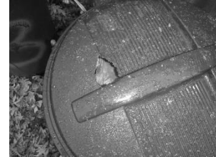
A lid with holes or cracks does not meet the requirement of a tight-fitting lid.
